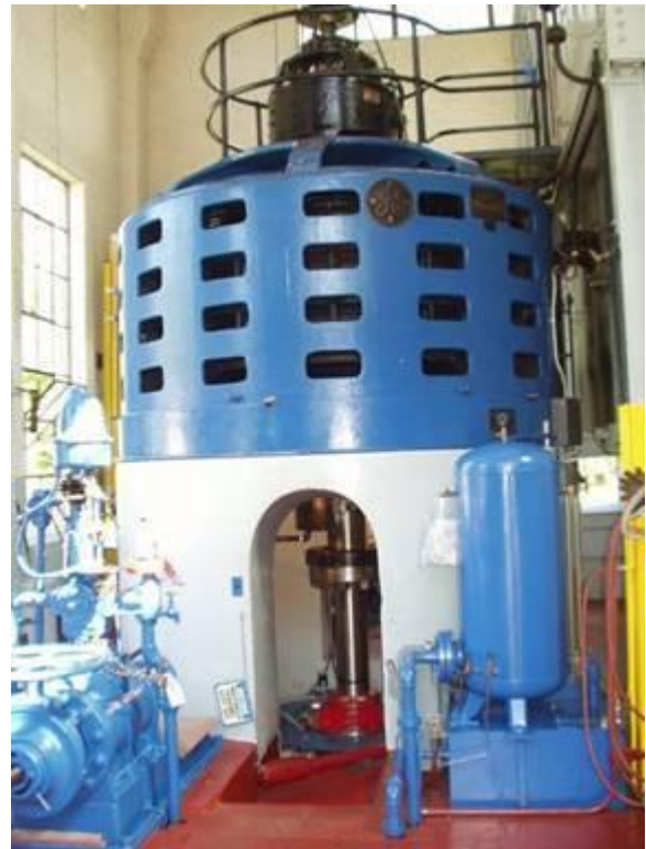
PHOTO 11 MARSHFIELD REFURBISHED TURBINE
