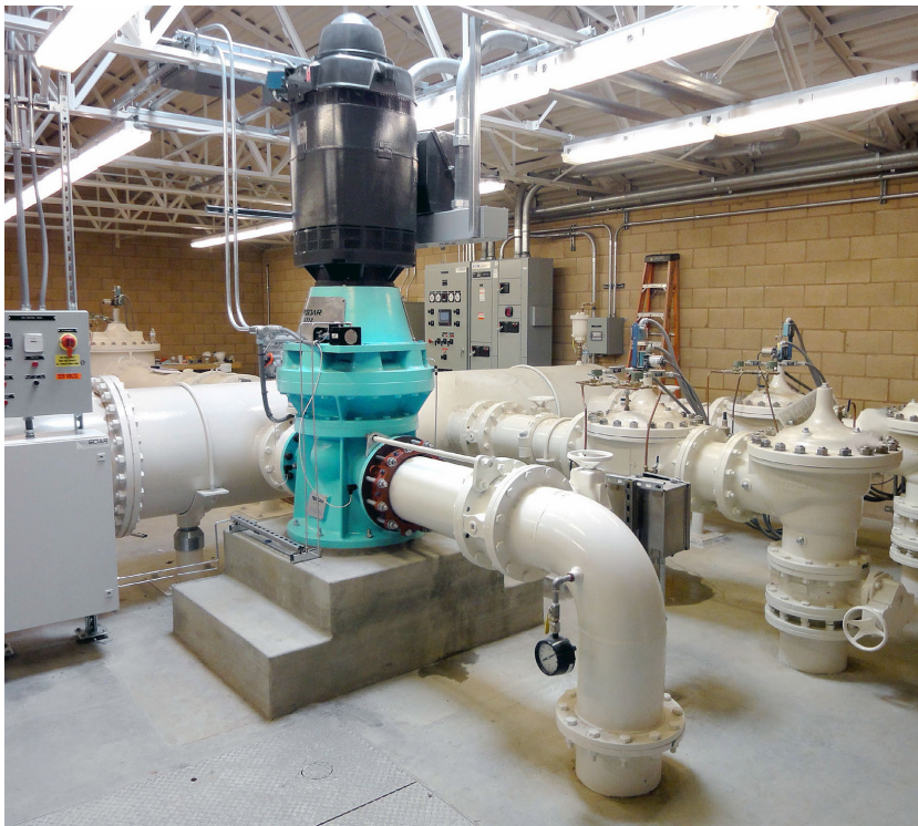
This is an example of a small conventional hydroelectric system. Photo courtesy of Canyon Hydro
